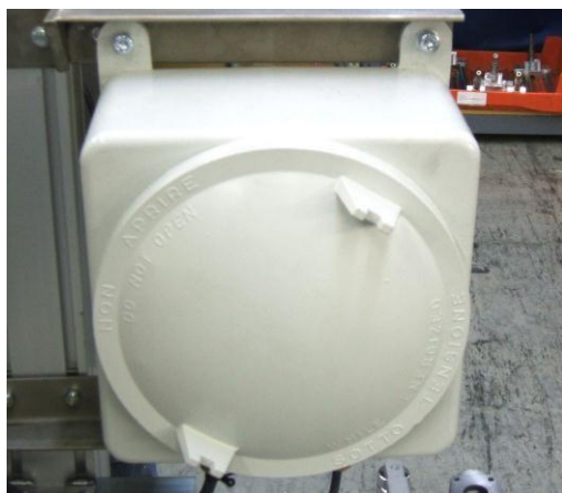
Battery and Charger Panel
